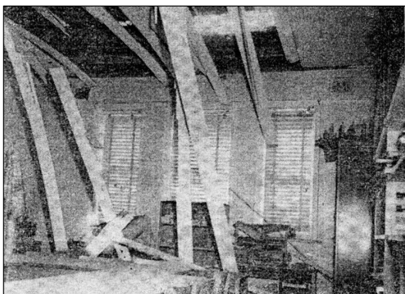
Some of the mess pupils and teachers at Robertson Public School had to contend with when they returned from their holidays on Tuesday. A falling chimney caused this damage, and a stone wall also collapsed.
